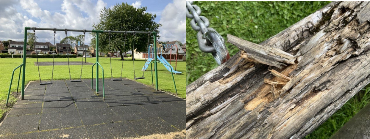
Example of Safety Flooring and Timber Activity Trails requiring replacement
